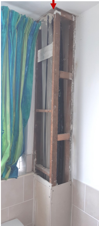
Soil pipe in a bathroom (with boxing removed)
