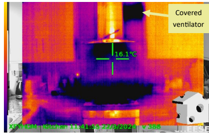
Ineffective closure lets in cold air
