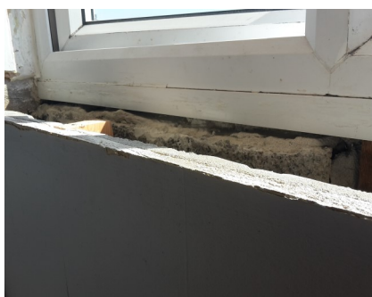
Gap between frame and masonry
