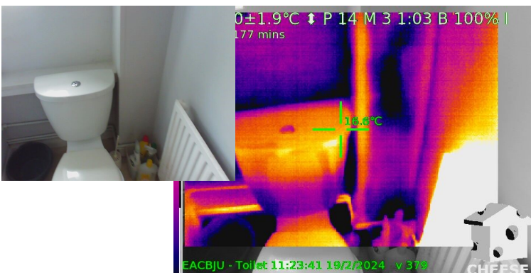
Cold patches on boxed-in waste pipe
