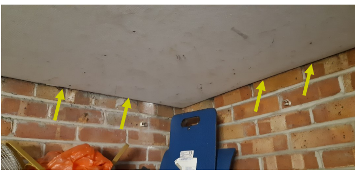
The ceiling board / wall gaps are not sealed
