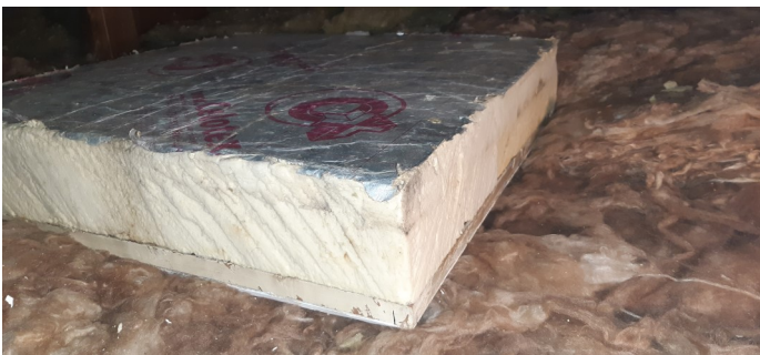
A well-insulated loft hatch with 100mm of Cellotex PIR insulation glued on with PVA adhesive
