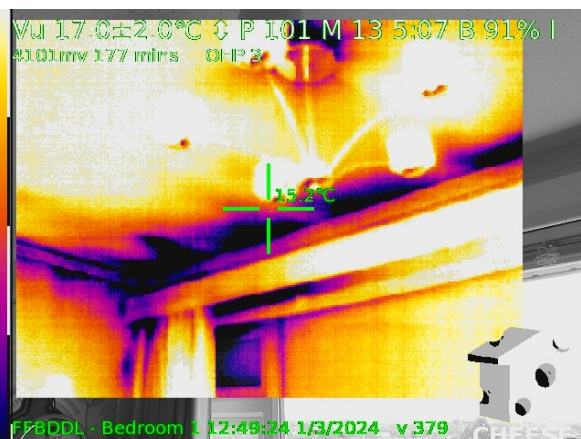
Cold eaves where insulation is too thin
